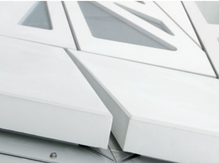
Casted fixing anchors
